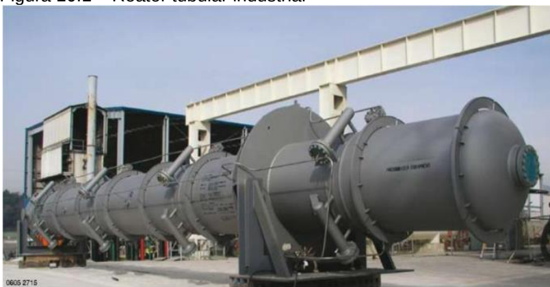
Figura 10.1 – Reator tubular industrial
