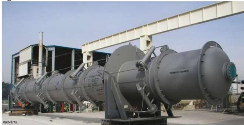
Figura 10.1 – Reator tubular industrial
