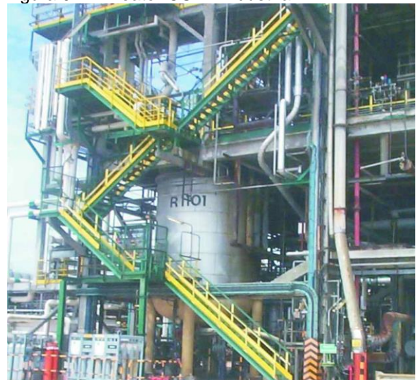
Figura 9.1 – Reator CSTR industrial
